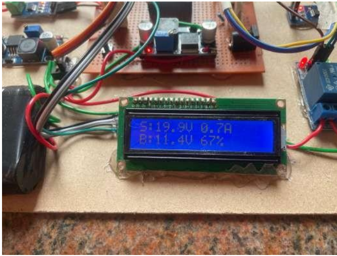
Fig. 4. LCD display of real time solar voltage, current, battery voltage and battery status.
