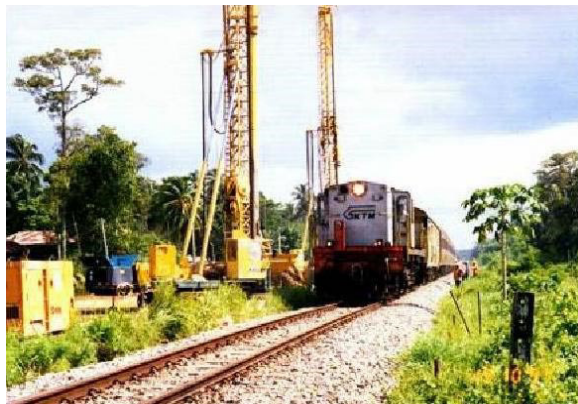
Fig.8 Vibro Replacement works along the KTM railroad line at Gurun for the Petronas Kedah Fertilizer Plant
